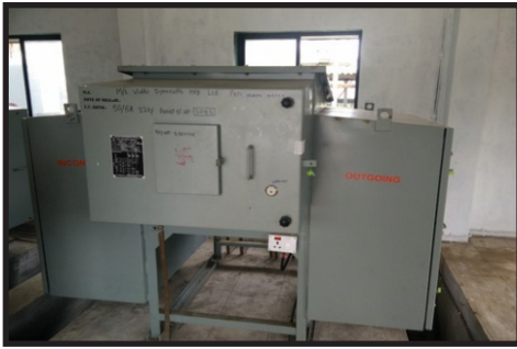
METERING KIOSK INSTALLATIONS
