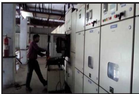
HT BREAKER SERVICING
