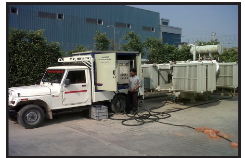
TRANSFORMER OIL FILTRATION
